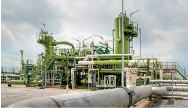
JT-LTS Plant and Condensate Stabilization Unit by Frames Netherlands
